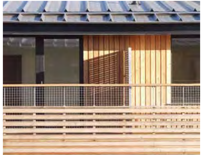
The layer of thinner horizontal boards are omitted at balconies to increase transparency
